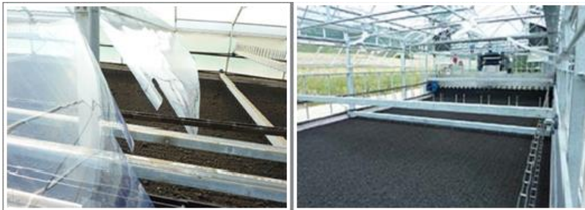
Fig: Solar Sludge Drying in Process
